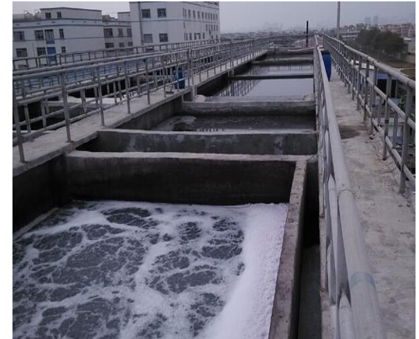
Tertiary Treatment for Re-use
